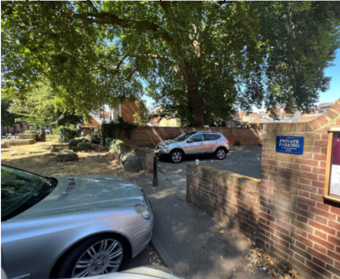
6. Photograph of existing half brick wall adjacent to St Mary's Church House
